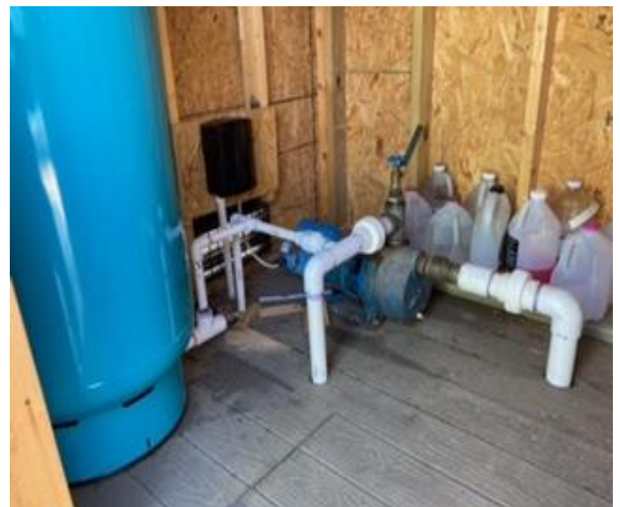
New tank connected to the pump
